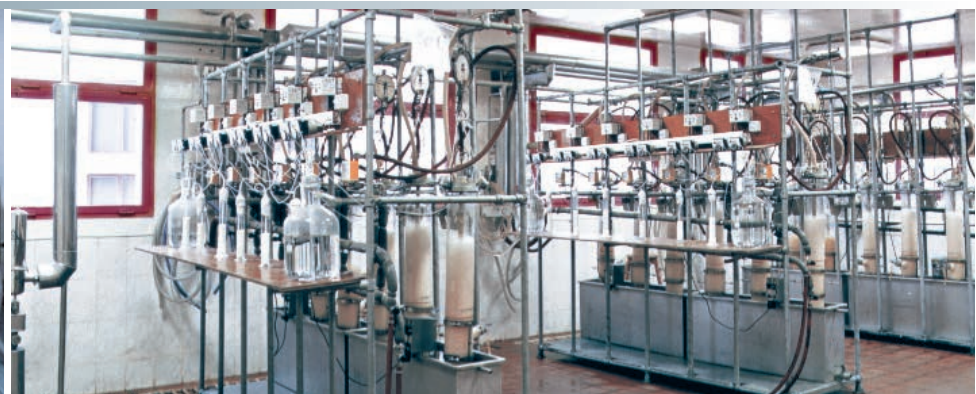
Pilot fermentation racks
